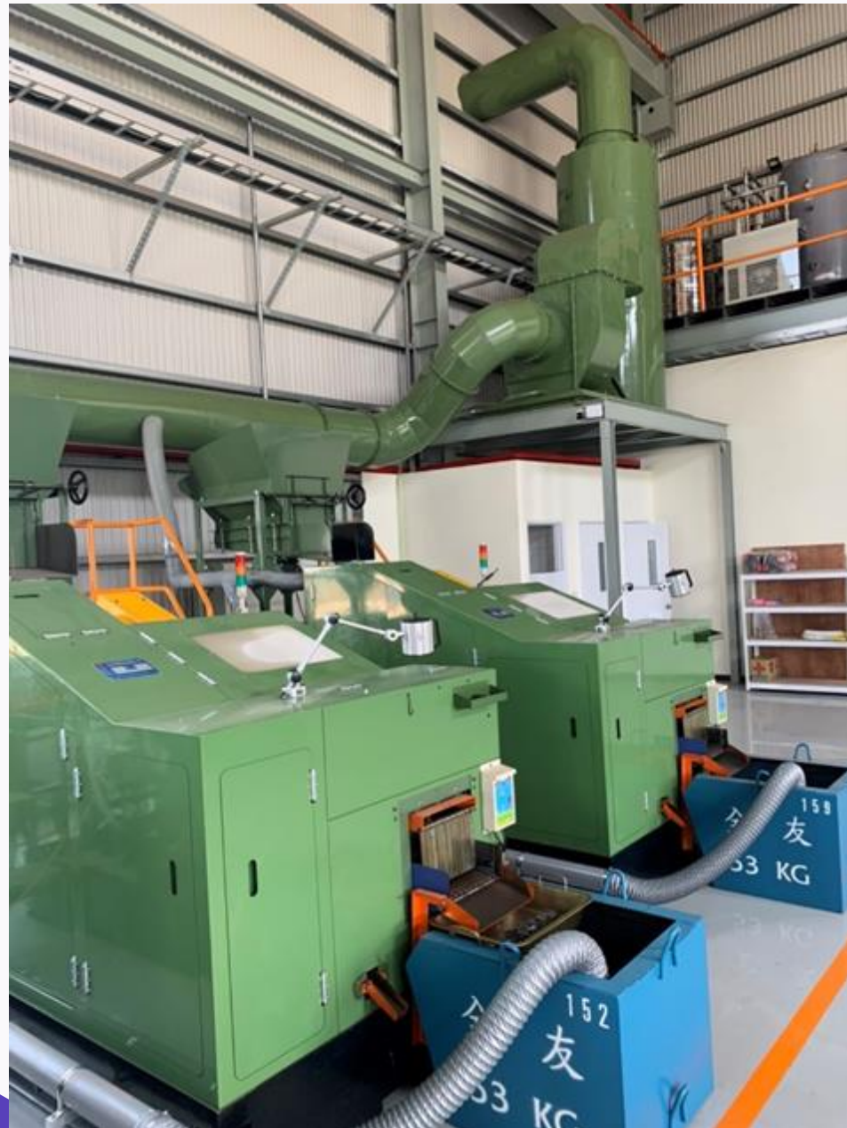
Dust collection Facility
